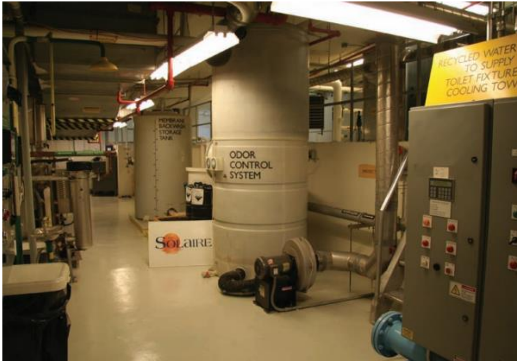
Figure 6 Solaire Wastewater treatment facility 5
