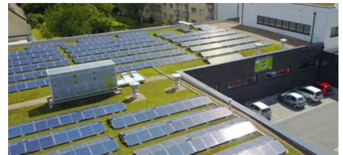
Figure 30: Rooftop Solar PV Systems
