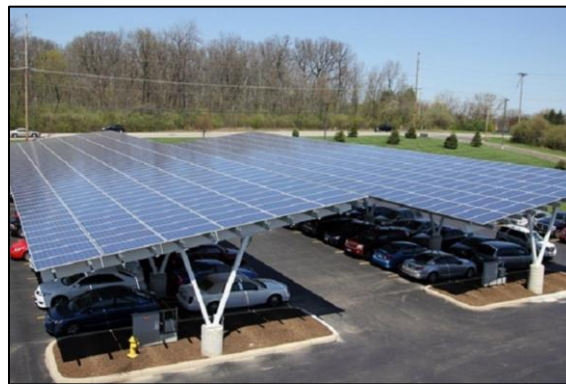
Figure 7: Carport PV System
